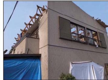
Photo 2 : a house damaged by Tornado
